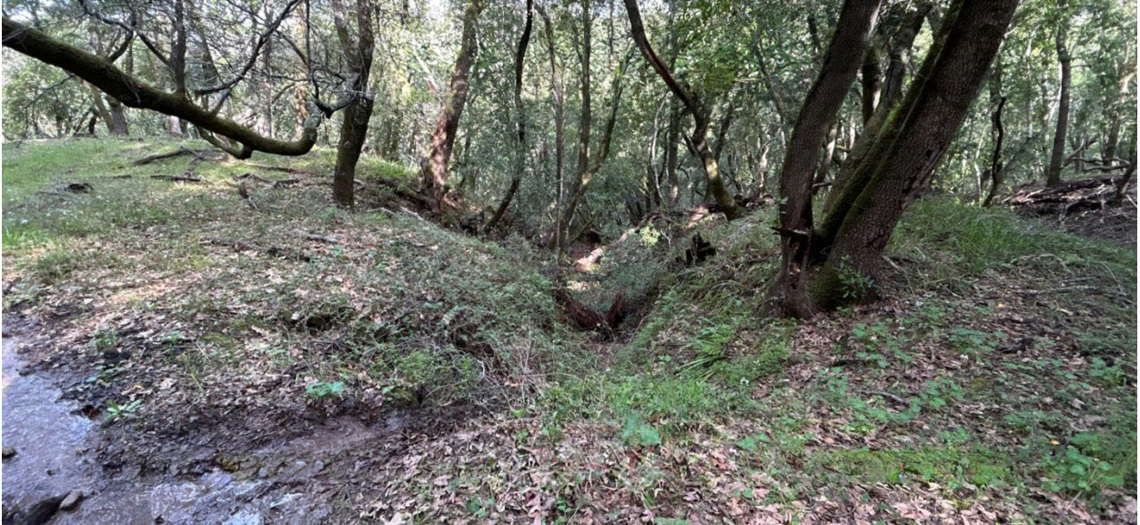
Photo 5. Road WB-02 looking down natural channel at OBF. Flows are being diverted down the left road approach instead of flowing into channel.
